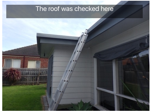
Rust to the high side of the roof sheets
